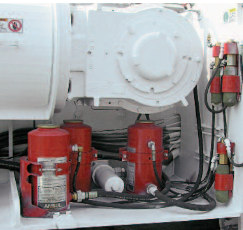
Fire Suppression System
