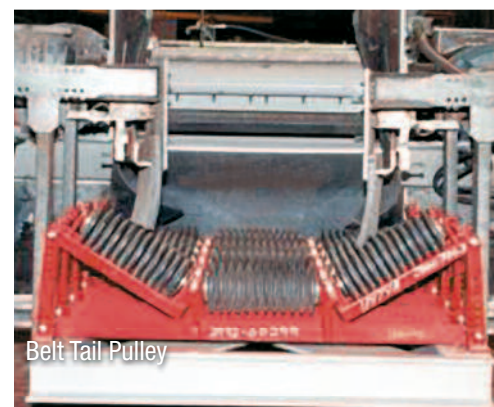
Breaker Roll Drive
